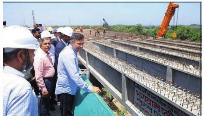
Verma said for the first time in India, a flyover has been designed with a dedicated cycling corridor
